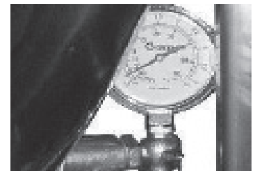
Each day confirm the jacket water level by checking the water gauge.
